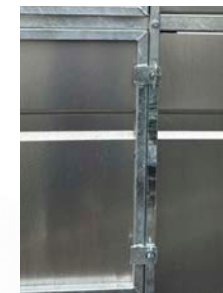
Two anti-luce pins on lower inspection door.
